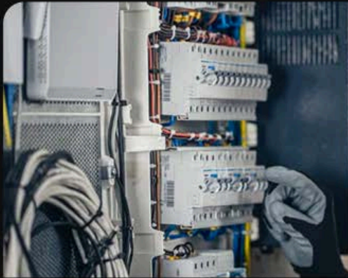
Electrical issues checking
